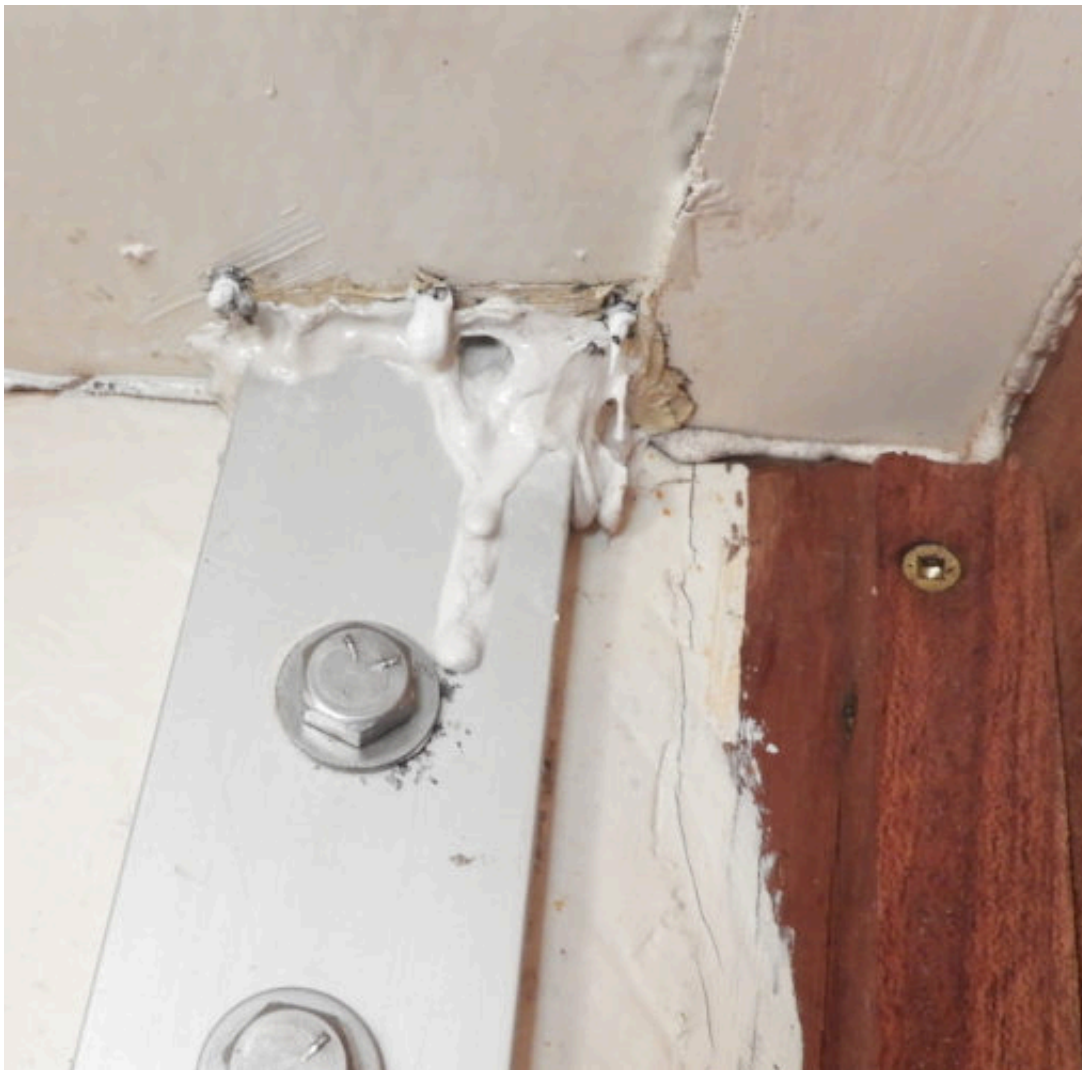
Chainplate with Butyl caulking drip
